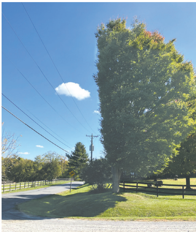
An example of a tree planted too close to a power line.
