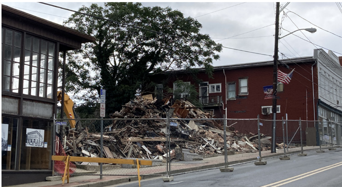
Demolition completed of fire-damaged buildings in the unit block of W. Potomac Street.
