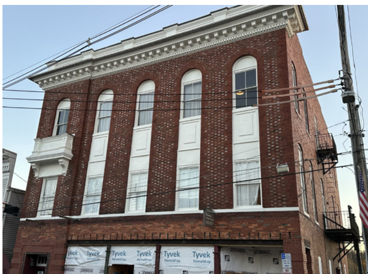
The scaffolding is gone from the front of the Brunswick Heritage Museum as renovations are nearly complete.
